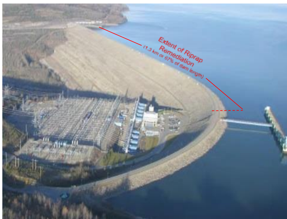
Figure 1 - Lateral Extent of Riprap Damage 5
